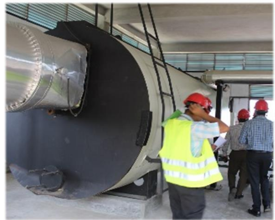
This efficient thermo oil heating system and exhaust gas boiler are saving 30,620 GJ of energy annually at an apparel factory.
