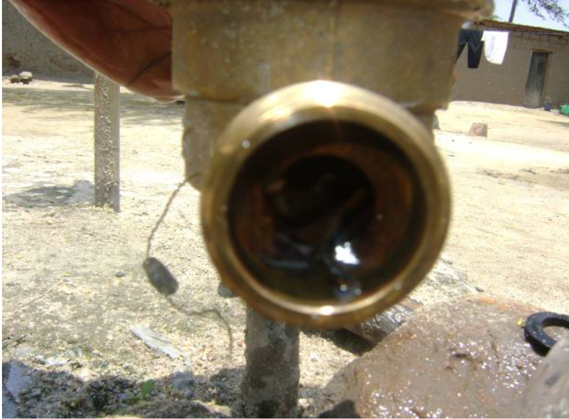
Figure 4: Meter with inserted steel wire to prevent it from measuring consumed water
