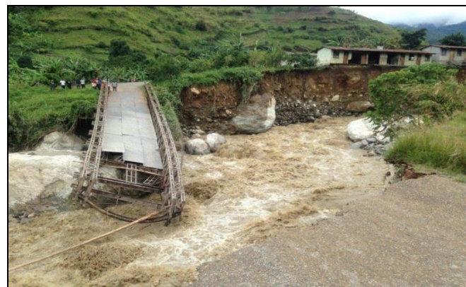
IMAGE 2. BRIDGE WASHED AWAY BY FLASH FLOOD, KASESE
